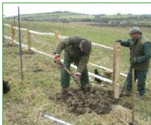
Oak post and riven ash rail fence being erected at Halstead by David Walker and Dave Barber.
