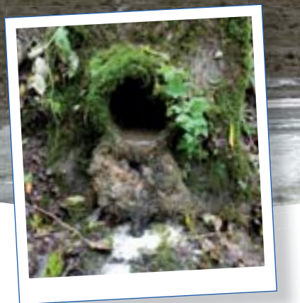
Surface run-off is clearly visible, but field drains flow more consistently.
