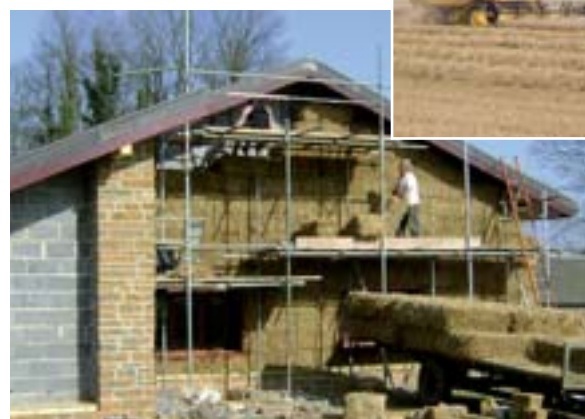
The wall insulation is constructed of straw bales made from the farm's own wheat straw.
